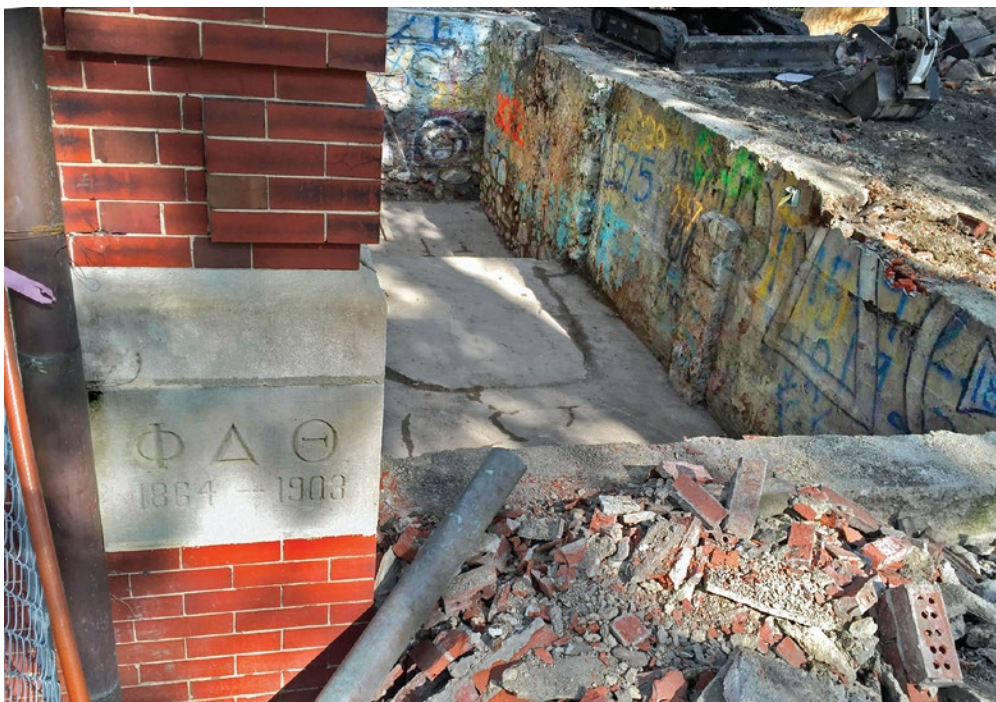
View of "The Bin" under the South Porch which has been completely removed as of early June. The cornerstone on the northwest side of the house is also visible.
